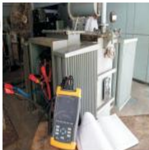
Energy & Harmonic Audit at 1000 KVA Transformer Secondary side
