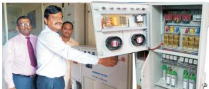
Three Phase Harmonic Filter for 20 KVA UPS
