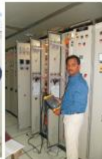
Energy Study and Harmonic Audit at VFD
