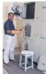
Harmonic Audit at M.V Panel ACB Incoming
