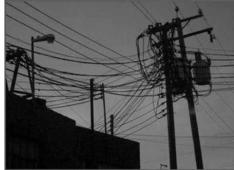
Fig.1 Transmission Line Connection with Wire
